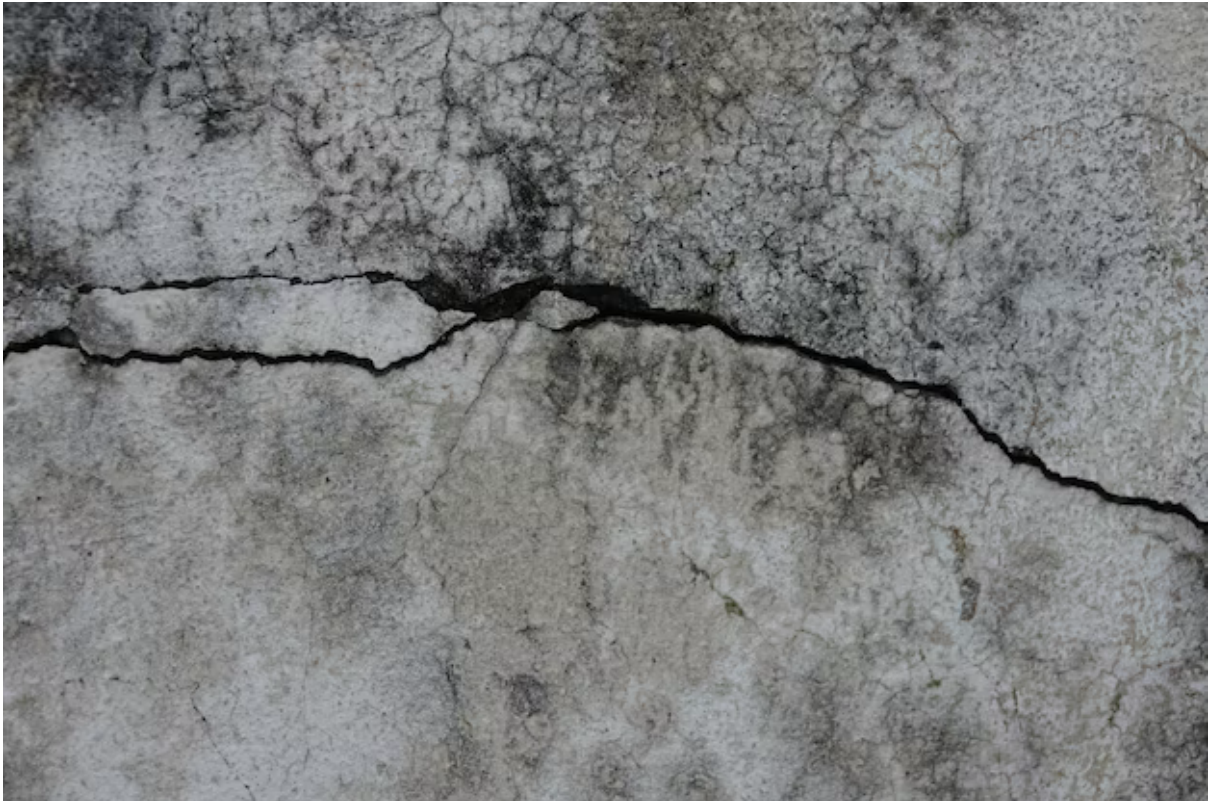
Cracks in concrete. [Image courtesy Freepik, royalty free images]
